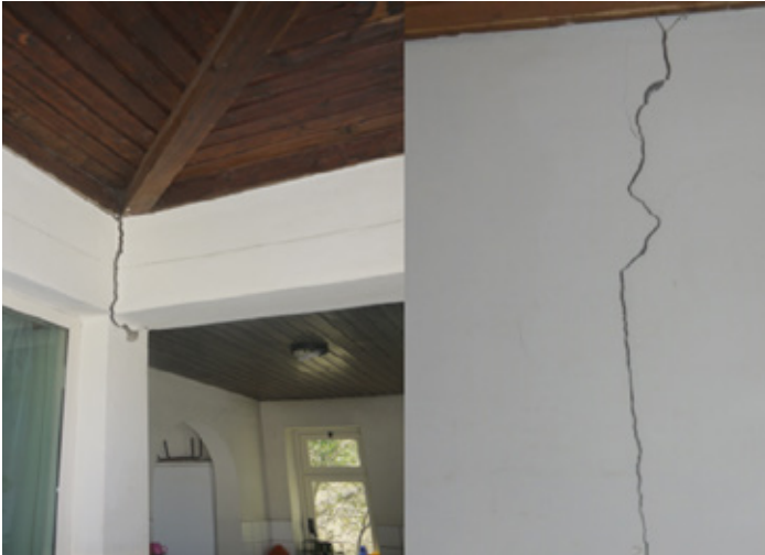
Cracks in SOS Family house
